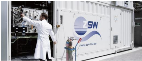
Figure 13 - View inside the research alkaline electrolyser of the ZSW.
